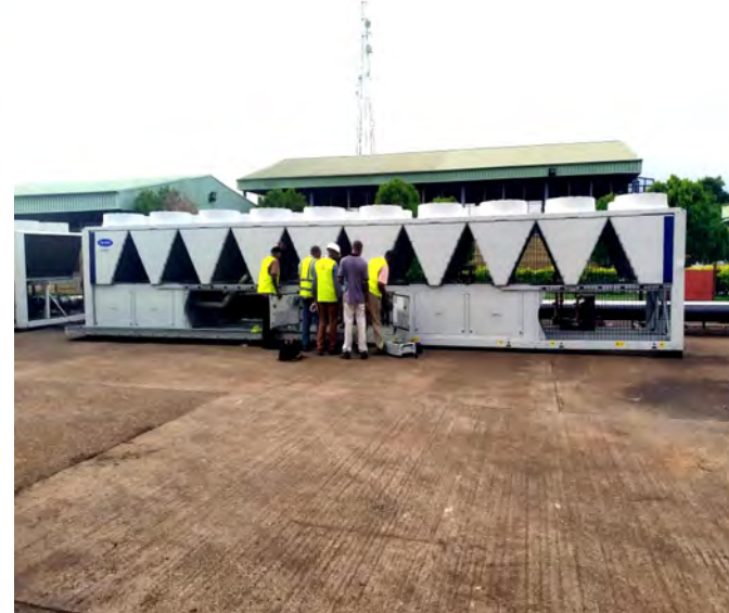
400 Tons Chiller at Cadbury PLC. Head Office
