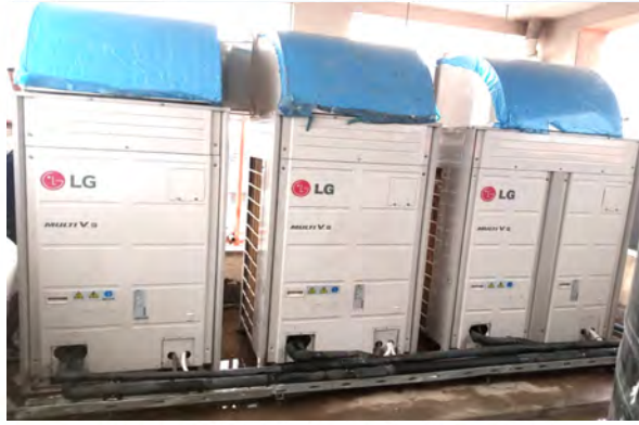
VRF System at FIRS Egbeda Lagos
