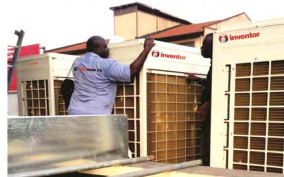
VRF System at Ogudu Mall
