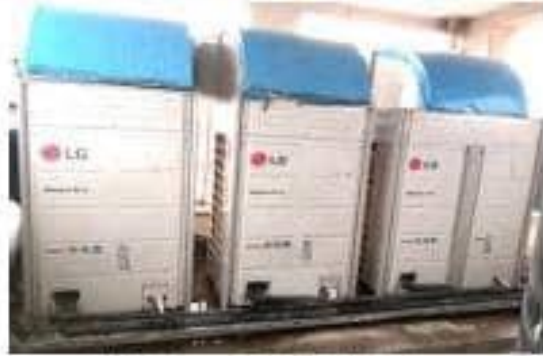
VRF System at FIRS Egbeda Lagos
