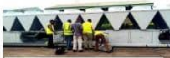
400 Tons Chiller at Cadbury PLC. Head Office
