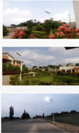
•Solar Street Lights.
