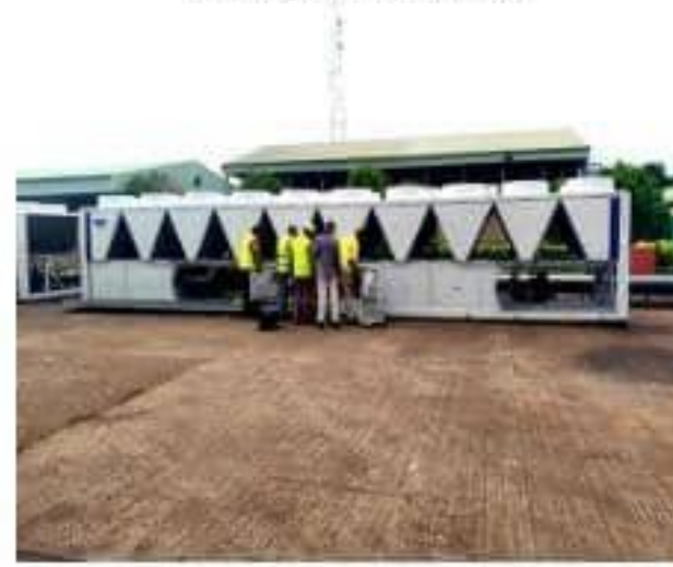
400 Tons Chiller at Cadbury PLC. Head Office
