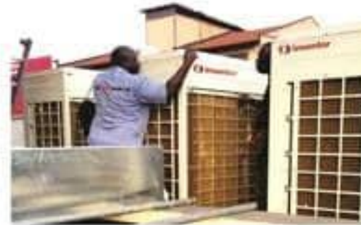
VRF System at Ogudu Mall
