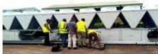
400 Tons Chiller at Cadbury PLC. Head Office
