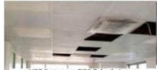
VRF System at FIRS Egbeda Lagos
