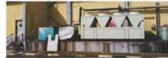
Chiller at Ondo
