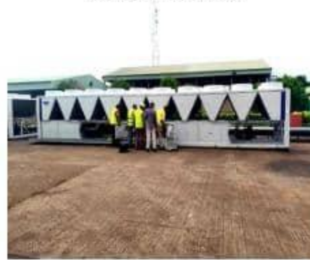
400 Tons Chiller at Cadbury PLC. Head Office
