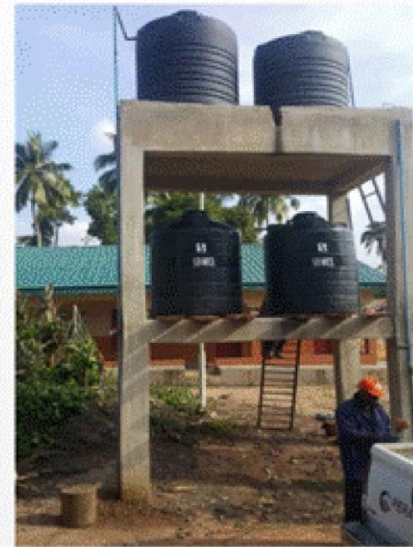
•Solar Water Pump.
